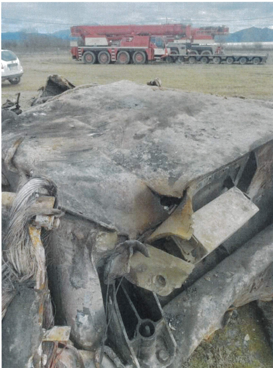
Figure 16: Transformer 120023 with explosion hole - file: 230307_123509.jpg
