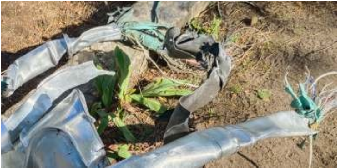
Figure 36 - Characteristic feature of the X-101 - cloth insulation of wiring
