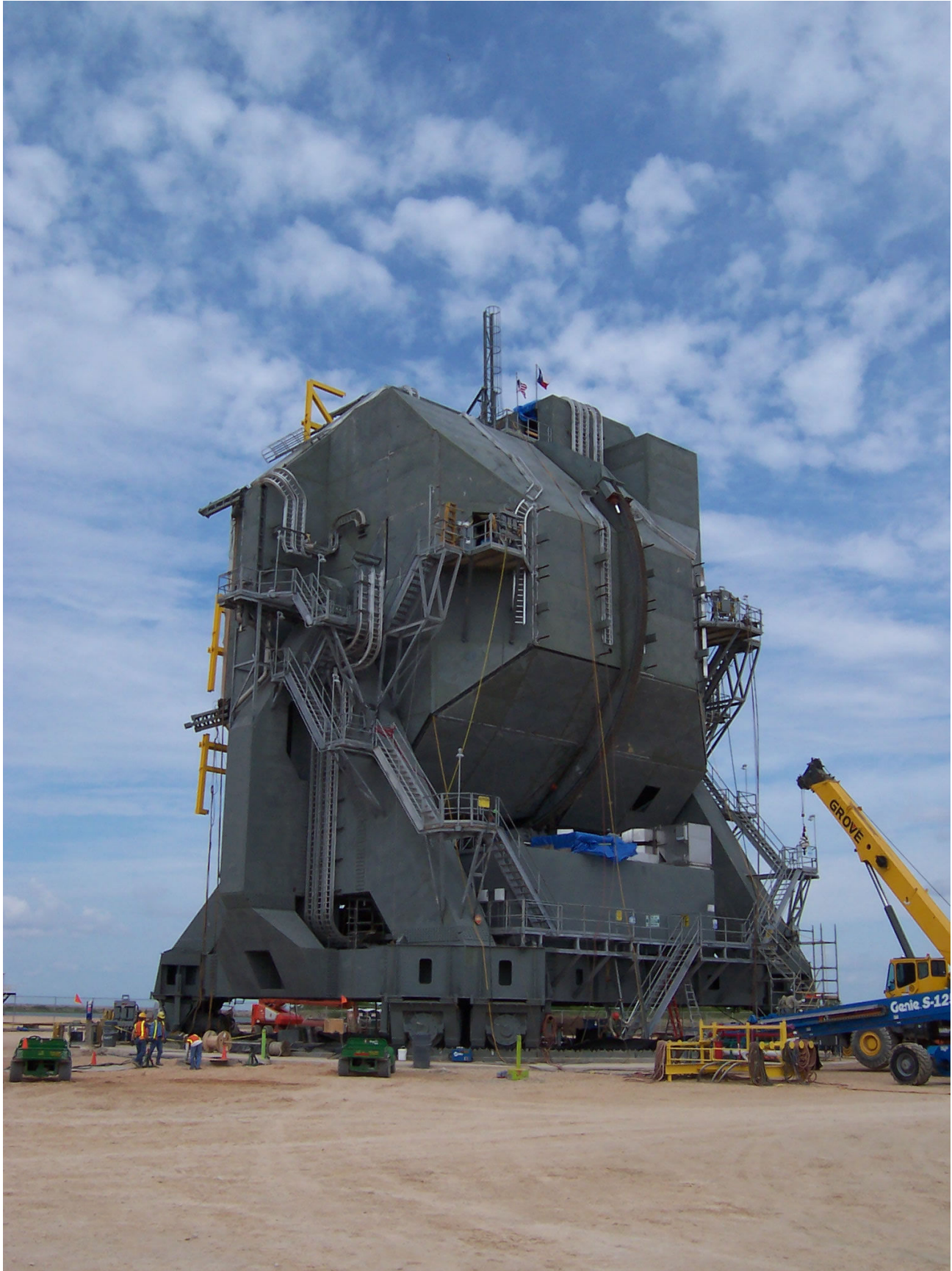
SBX radar mount at Ingleside
