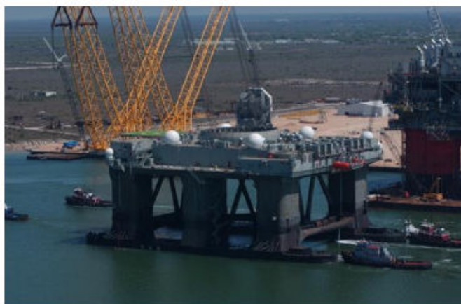
The Sea-Based X-Band Radar platform arrives at Kiewit Offshore Services in Corpus Christi, Texas on March 17, 2005. While at Kiewit, the 2,000 ton X-Band Radar (seen directly behind the platform) will be lifted onto the platform later this spring.
