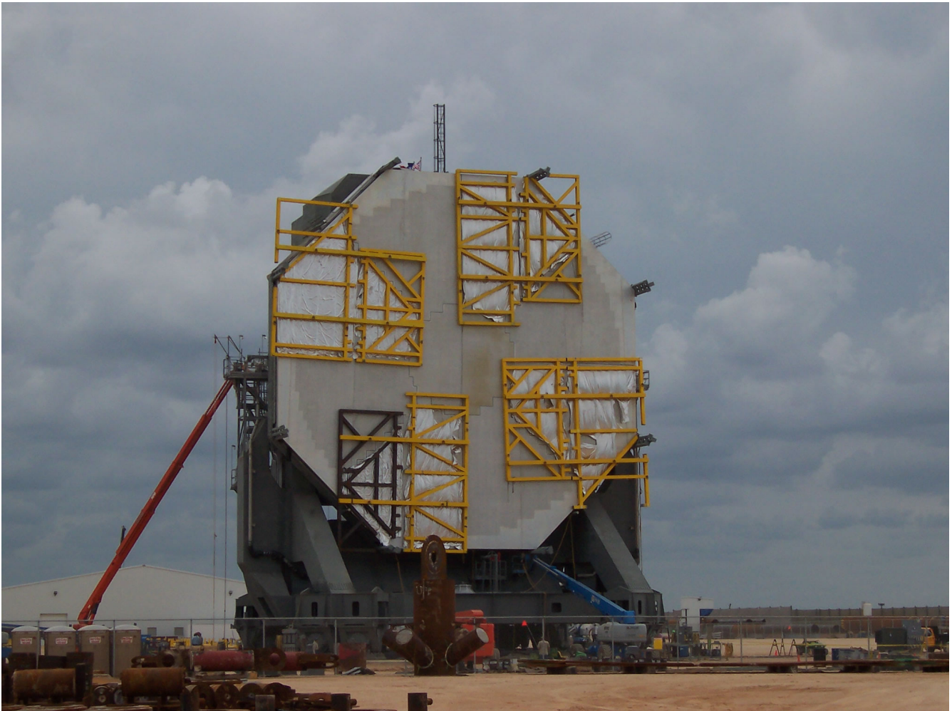
SBX radar mount at Ingleside
